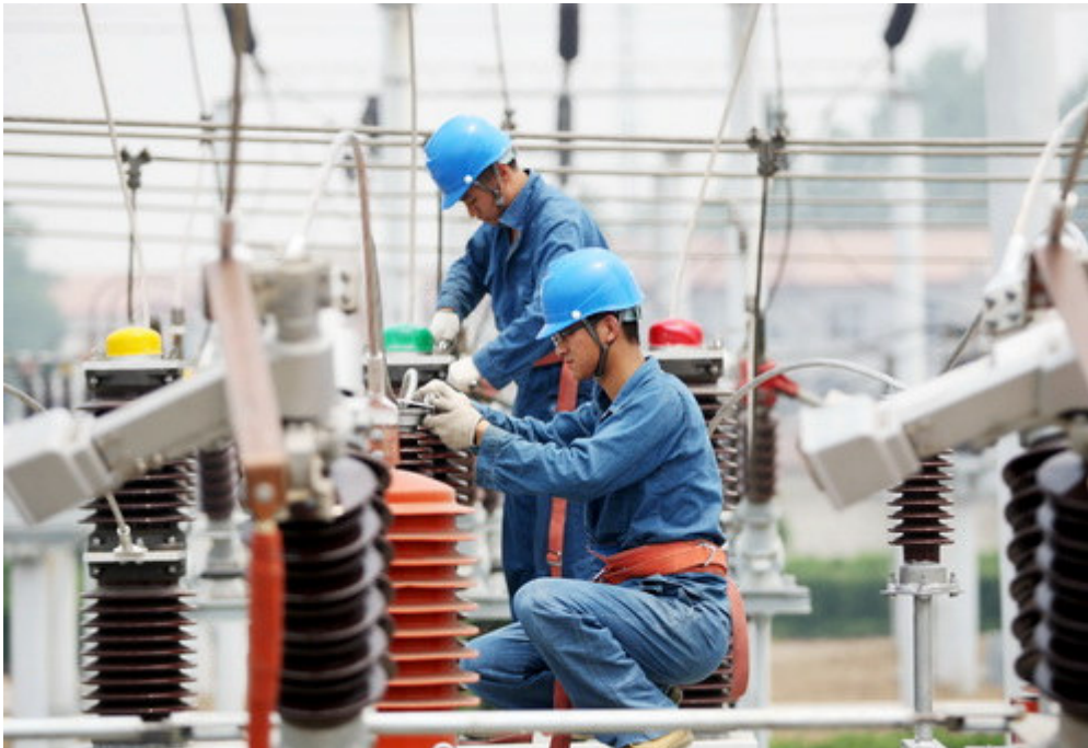
Workers carry out maintenance work at a power installation in Anhui province.
